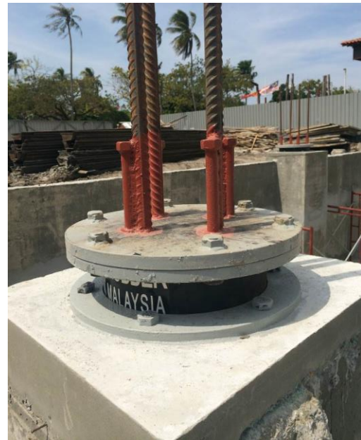
Figure 9 Bearing mounted on a concrete pedestal
