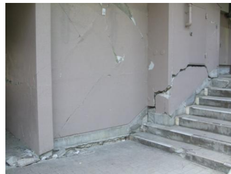
Photo 3. Damage caused by the different height of the first storey
