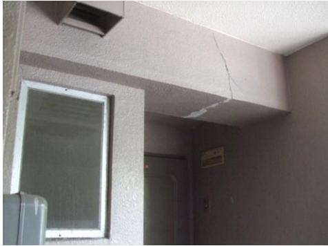
Photo 4. Crack of the girder of the second floor
