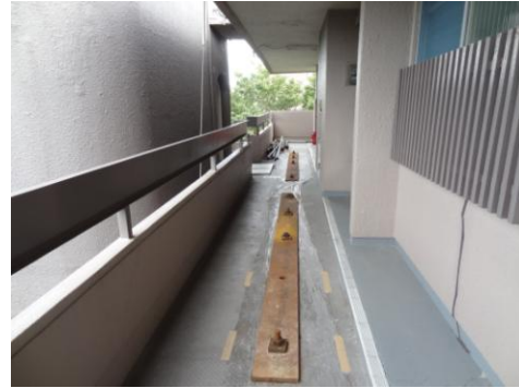
Photo 5. Temporary reinforcement of the east edge of corridor of the second floor
