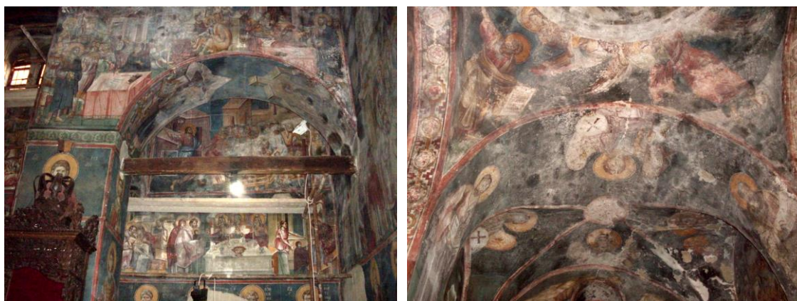
Figure 3. Existing cracks in the church repaired in 1986
