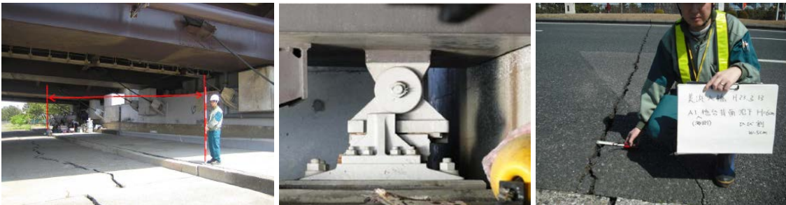
Figure 1. Observed cracks, settlement, and lateral spreading after 2011 Great East Japan Earthquake at the Mihama Bridge in Chiba City, Japan (Chiba City 2011)
