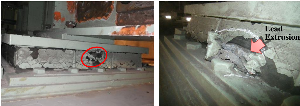
Figure 5. Damage status of lead extrusion
