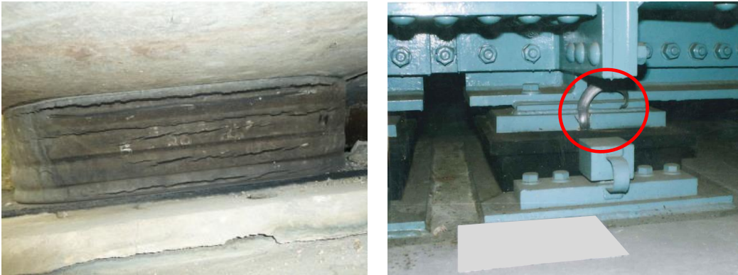
Figure 2. Damage examples of rubber bearing (Left : Crack, Right : Lead extrusion)
