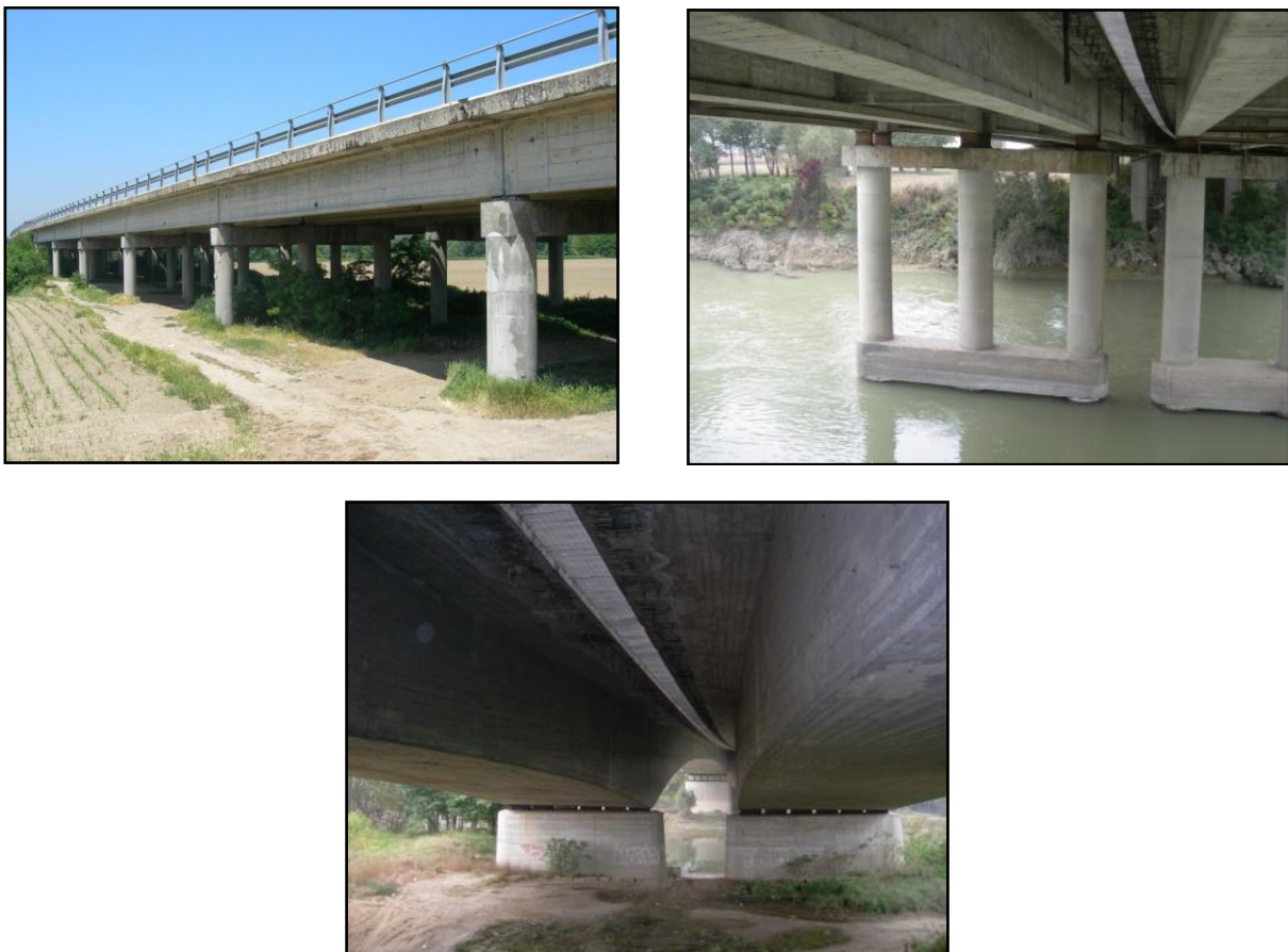
Figure 1. Bridge over the Tanaro and Bormida rivers: r.c. beam deck (top-left), p.c. beam deck (top-right) and box girder deck (bottom).
