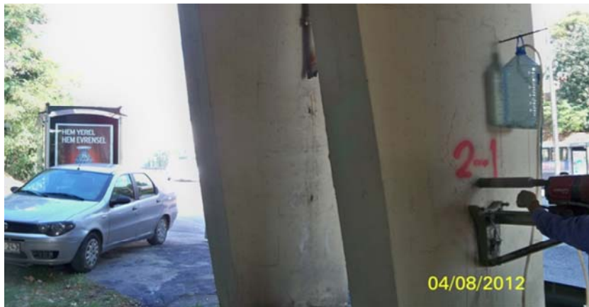
Figure 2.7. Extraction of concrete core specimens from the pier for material quality test (Üsküdar-Haydarpaşa Overpass Bridge)
