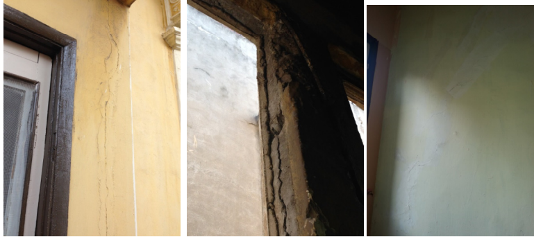
Figure 2. The photos of the building elements showing some bending and shear cracks.
