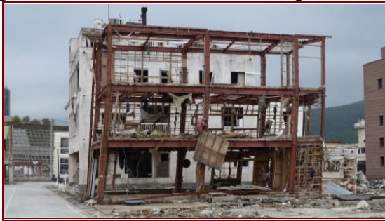
Figure 3: Global lateral deflection/failure due to lateral fluid load (hydrostatic and hydrodynamic) (EEFIT 2011).
