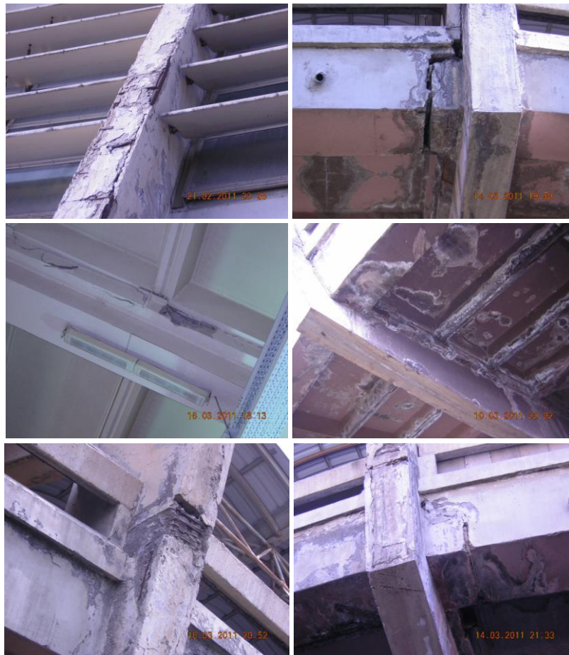
Figure 3. Damages of the reinforced concrete members
