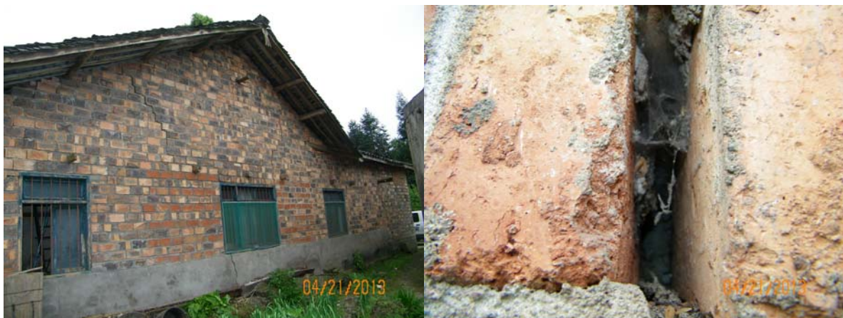
Fig.4 A rural building with poor seismic resistance property in intensity VI area in south of Lushan earthquake epicentre. The spider web and dusts on it indicated that the cracks in the brick load-bearing wall were not directly damaged by the Lushan earthquake. The probably reason for these cracks were uneven settlement of foundations before the event, which were very common in mountain areas of Western China.
