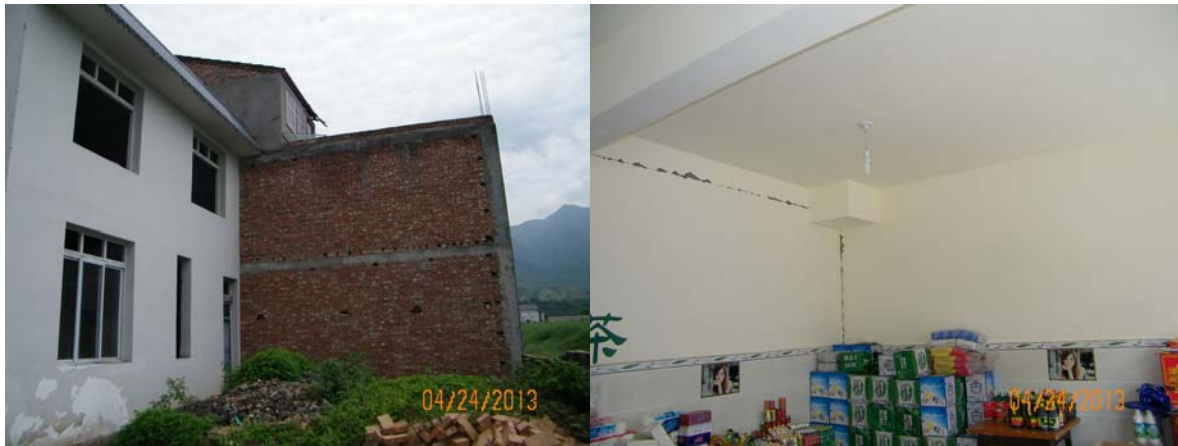
Fig.5 A rural building with high seismic resistance property in intensity IX area in the rebuilt area of Wenchuan earthquake, whose filler walls cracked but load-bearing walls and beams were undamaged.
