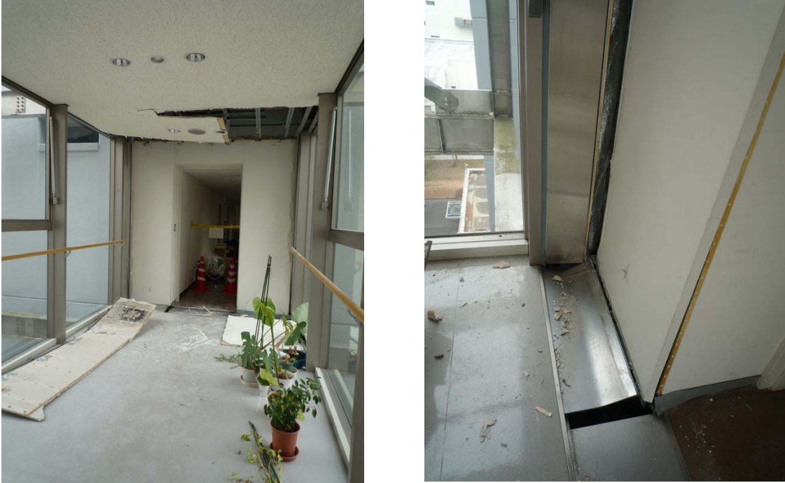
Figure 8. Damage to the expansion joint and passageway at the eighth floor
