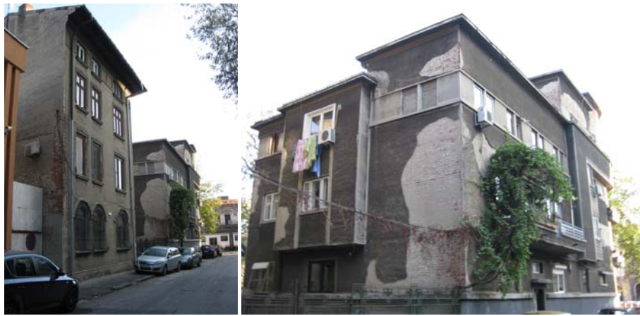
Figure 6. Reinforced concrete and masonry mid-rise residential buildings of the 1930's proving lack of maintenance (Photo E. S. Georgescu)
