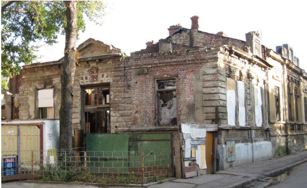
Figure 4. Masonry houses that resisted earthquakes but are now threatened by lack of maintenance, as the ownership situation and financial ability are at stake on Str. Justiției (Photo E. S. Georgescu)
