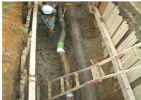
Figure 1. Upheaval buckling of 4” pipe
