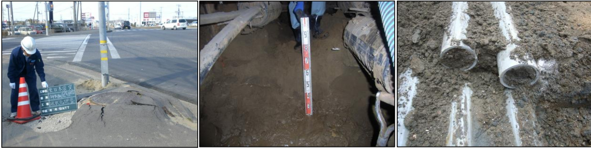
Figure 3. Damaged cases of telecommunication infrastructure in the liquefaction area
