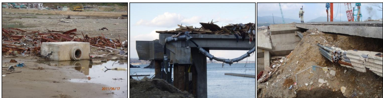
Figure 2. Damaged cases of telecommunication infrastructure in the tsunami area
