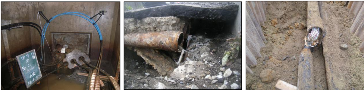
Figure 4. Damaged cases of telecommunication infrastructure in the other area
