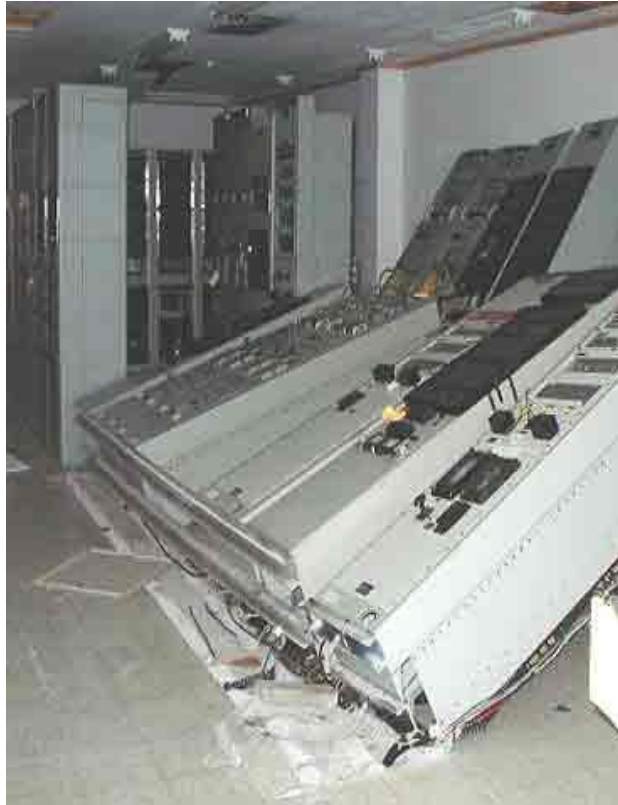
Figure 8. Photo of electrical panel failure caused by earthquake lateral forces.
