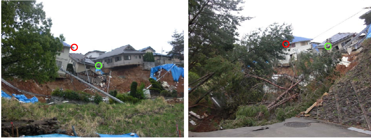
Photograph 1. Damage condition at the slope site of interest based on the author's reconnaissance results
