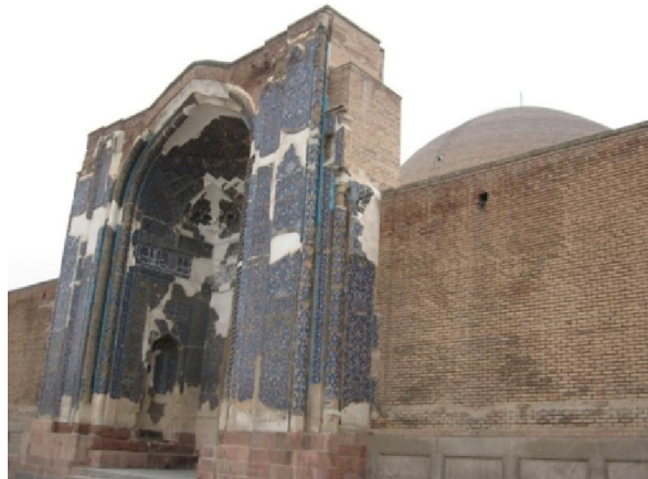
Figure 2. Damages to Kabood Mosque by the Tabriz, Iran Earthquake of 1778
