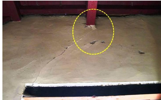
Figure 22. Improper connection of roof beam and wall
