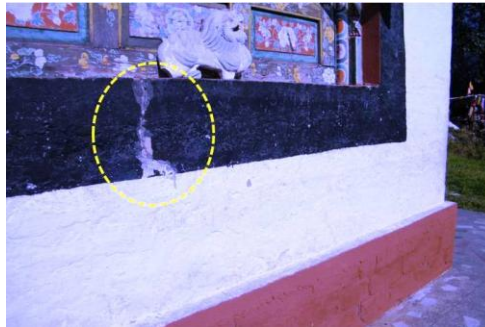
Figure 18. Vertical crack on sill
