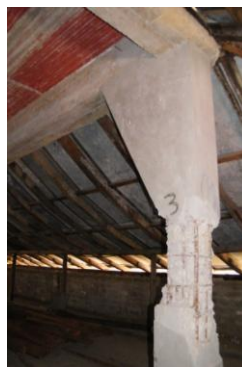
Figure 14. Poor column - beam joint
