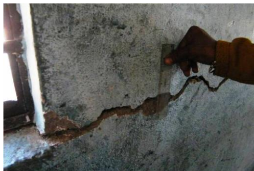
Figure 19. Horizontal Crack on sill level
