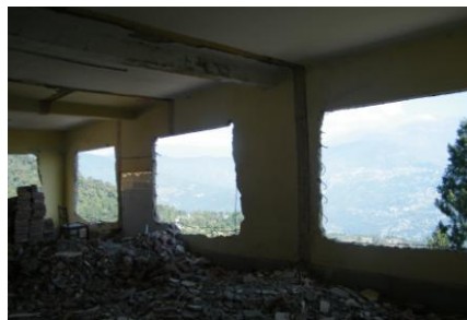
Figure 7. Collapse in the wall
