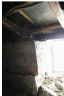
Figure 13. Collapse of random rubble stone masonry wall at top floor
