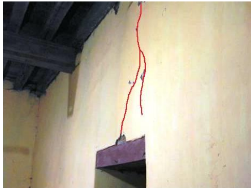
Figure 10. Crack on spandrel masonry
