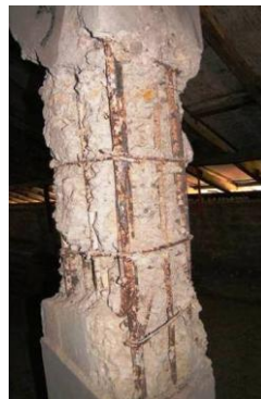
Figure 16. Spalling of concrete
