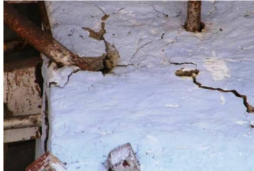
Figure 12. Cracks on wall masonry
