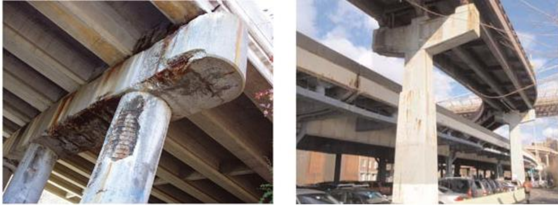
Figure 3: Corroded bridge piers (Akiyama and Frangopol 2013, Ou, Fan et al. 2013)
