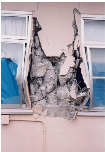
Damage class V:
