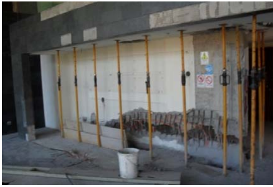
a) Wall with compression damage, 17-story, mixed-use building constructed in 2009, Chile (Moehle 2012).
