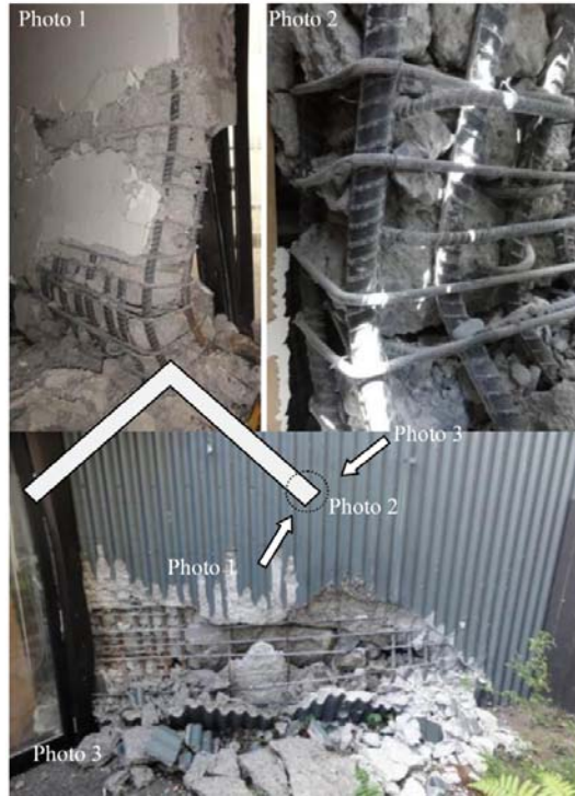
c) Wall with compression damage, 7-story commercial building, Christchurch, NZ (Kam et al. 2011).
