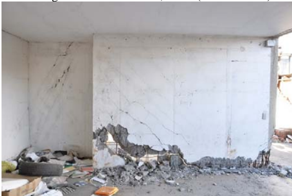
b) Wall with compression and shear damage, 12-story residential building constructed in 2006, Chile (Moehle 2012).
