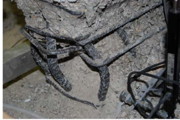
b) Compression damage in boundary element of slender wall test specimen PW4 shown in a).
