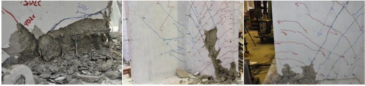
The first failure mechanism
