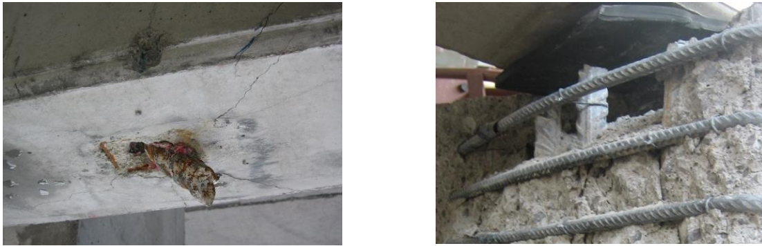
Figure 2. Local ductile failure and global failure of a dowel connection
