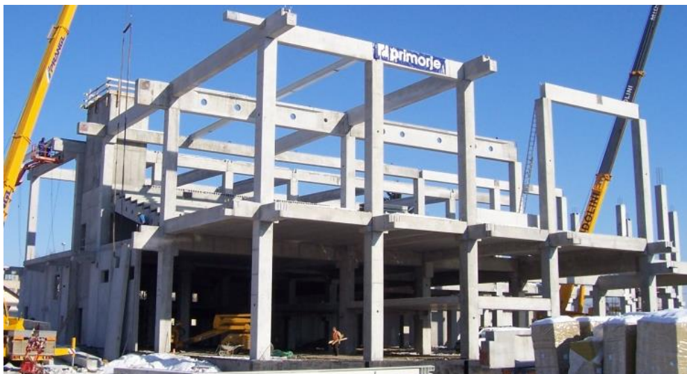
Figure 1. The most common structural system of precast industrial buildings in Europe consists of an assemblage of slender cantilever columns, tied together by beams.
