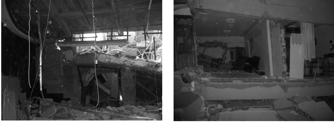
Figure 1. The photos of the severely damaged buildings caused by the 2011 Van (Turkey) earthquake; taken from a) a commercial building, b) a residential building (courtesy of Murat Ayhan)
