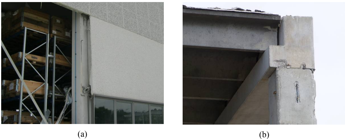
Figure 4 Failure of cladding panels: a) failure due to the light connections, b) tensile failure of the steel fasteners (both left and front sides)
